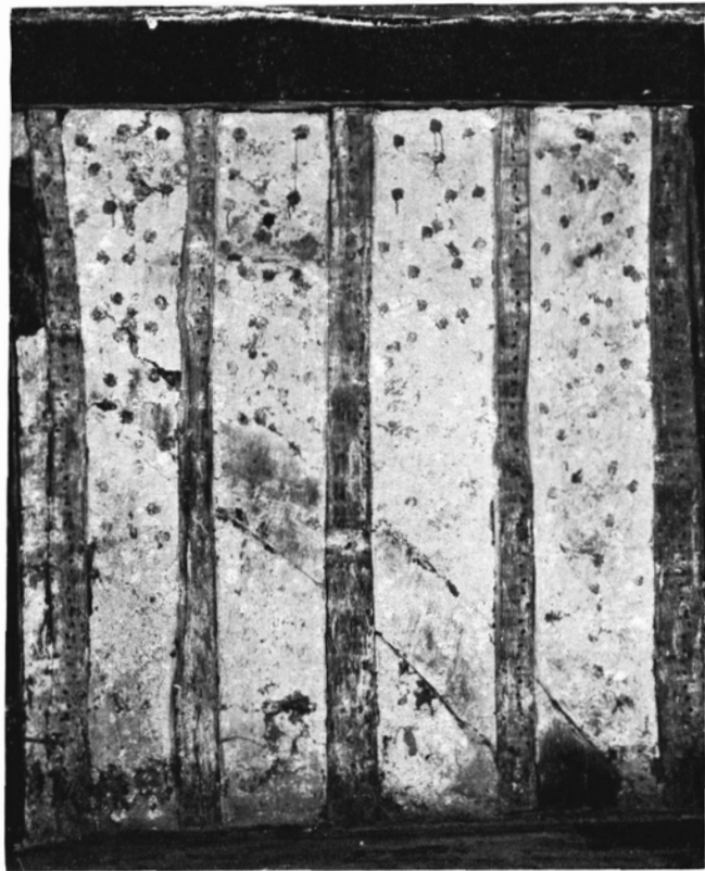
B. Decoration on limewashed Daub Filling between Studs in lower half of Partition shown in Plate IB.
